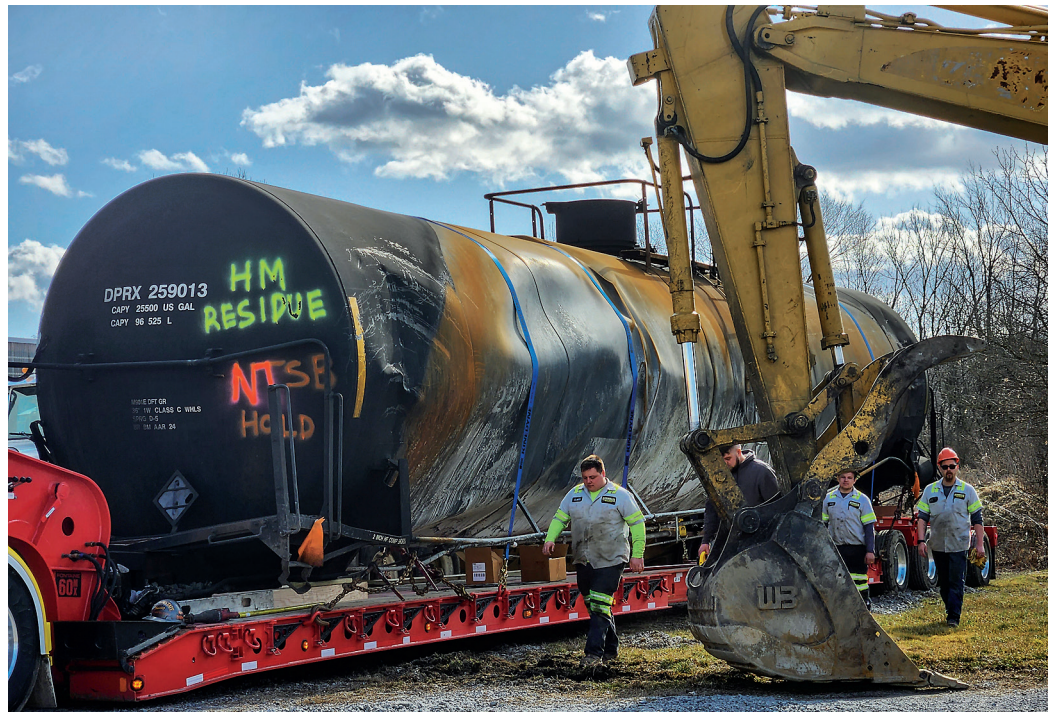
(Above) Heavy load trucks haul away freight cars that were damaged in the Feb. 3 Norfolk Southern Railway derailment in East Palestine, Ohio. (Top Middle) Drone footage shows the freight cars on fire on Feb. 4. (Bottom Middle) The continuing cleanup of portions of the Norfolk Southern freight train on Feb. 7.
