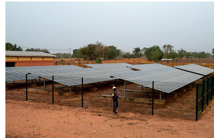
Solar panels installed in the Takpapieni village, Togo, on Feb. 14, 2020.
