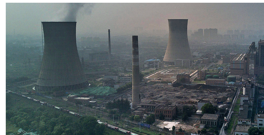
A Chinese state-owned coal-fired power plant in Huainan, Anhui Province, China. The Chinese Communist Party built more than three times as much coal-power capacity as the rest of the world combined in 2020, according to a report.
