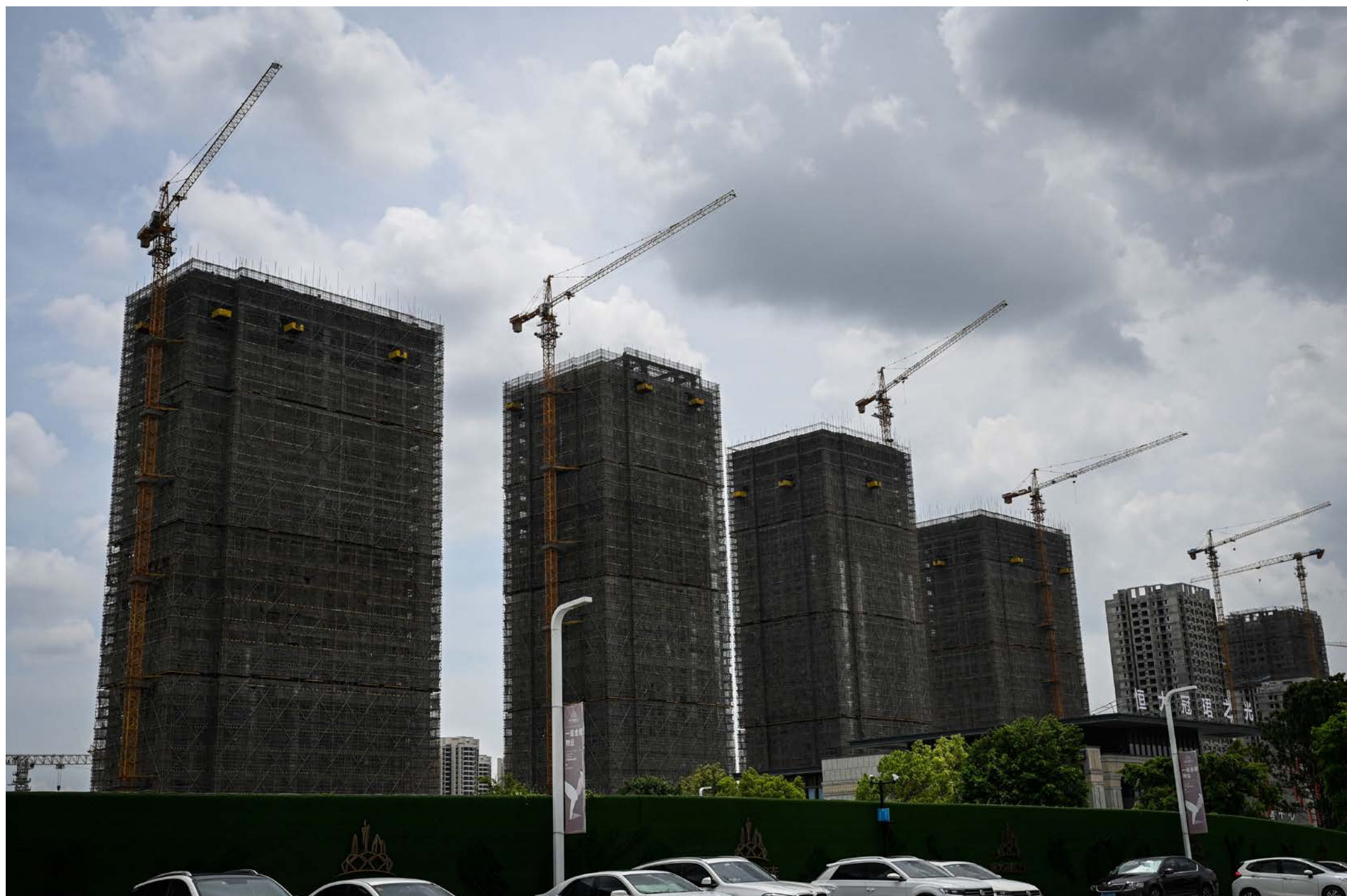
Evergrande residential buildings under construction in Guangzhou, Guangdong Province, China on July 18, 2022.
