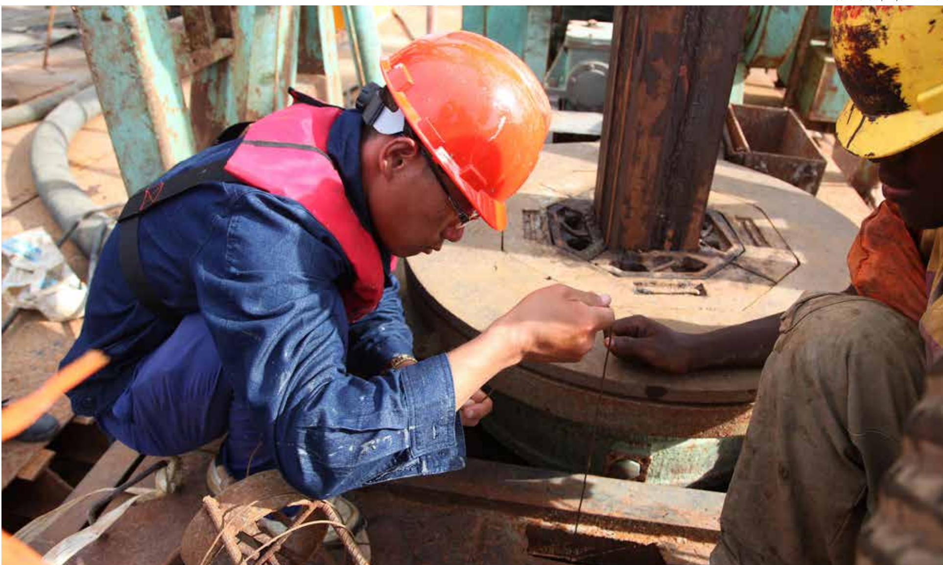
A technician with a Chinese company works at the construction site in Dar es Salaam, Tanzania, on March 23, 2013.
